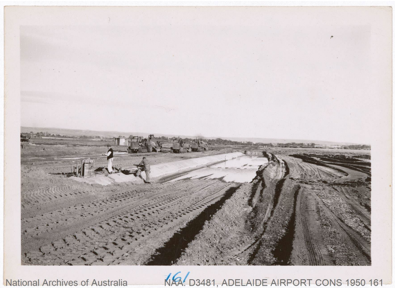
Figure 3 – Adelaide Airport early 1950's - during construction - flooding of sandfill in trench prior to compaction 28 July 1950 – NAA D3481, ADELAIDE AIRPORT CONS 1950 161
