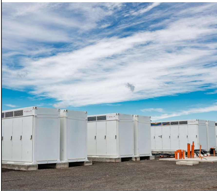
Figure 7 - photo of Tesla Megapacks installed on raised foundation pads
